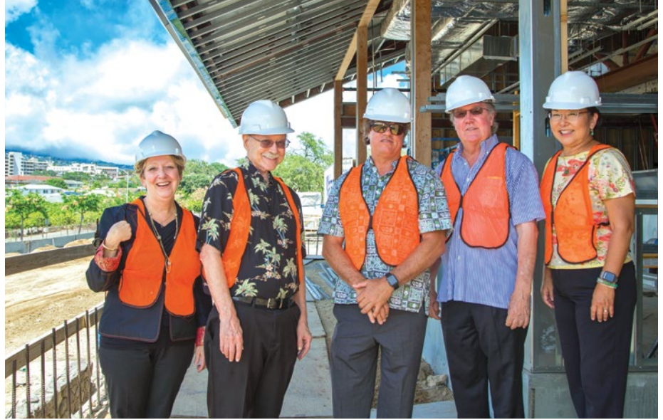
(L-R): Rebecca Smith, John Morton, Daniel Hilton, Noel Trainor & Mariko Miho tour the Culinary Institute of the Pacific construction site.
